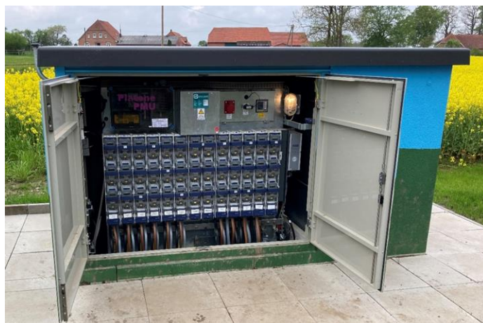
Figure 7: Smart secondary substation – low-voltage connection to bus bar
