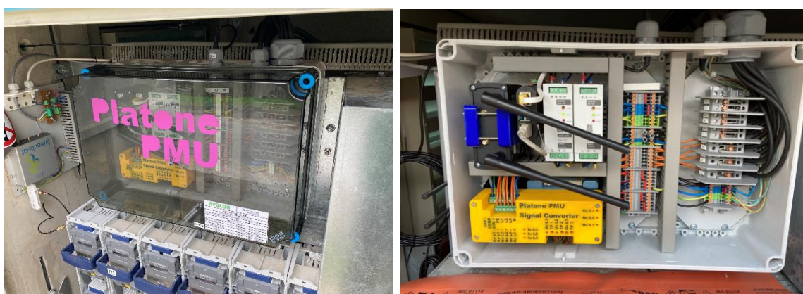
Figure 9: Phasor measurement unit with LTE communication device
